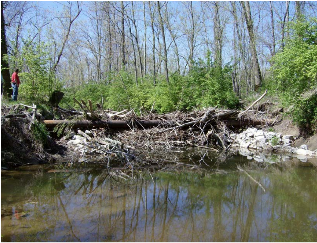
Snag at Braeswood Flyover on Engle Creek – 5/07
