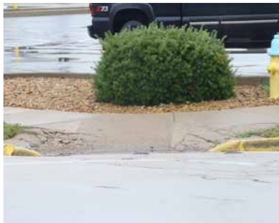
Right: A deteriorated handicap ramp located at the intersection of Lincoln and Third.
