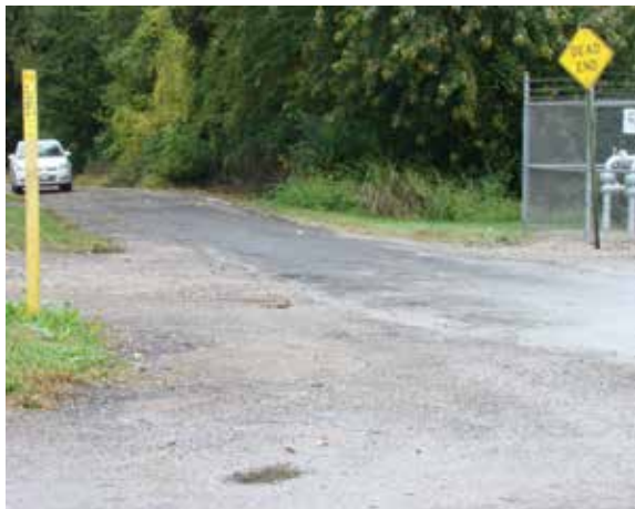
Left: Deteriorated pavements on W. First Street.
