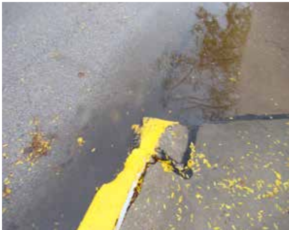
Left: Deteriorated curbing along Lincoln Avenue. Note: standing water due to inadequate storm drainage.
