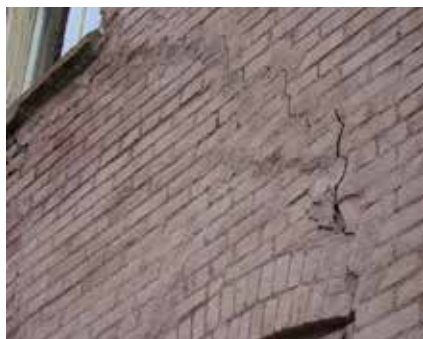
Above: Another example of the deteriorated brick wall at 2 S. Lincoln.
