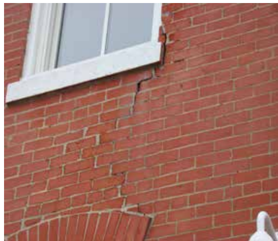
Right: A deteriorated brick wall at 226 W. State Street.
