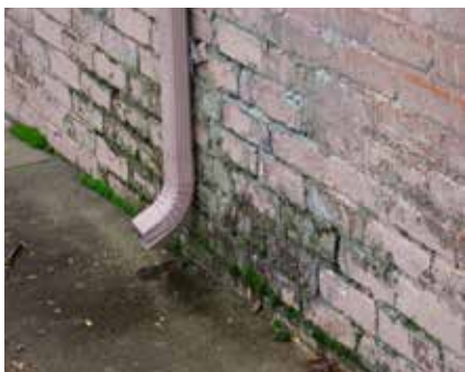
Above: The brick wall at 2 S. Lincoln Avenue is deteriorated.
