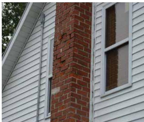
Left: The chimney on 229 E. State Street is deteriorated.
