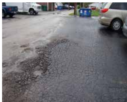
Above: A deteriorated parking lot located at 117 N. Lincoln Avenue. Note: un-screened dumpsters.
