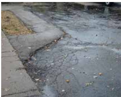
Below: The parking lot at 31 S. Lincoln Avenue is deteriorated.
