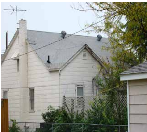
Left: 119 E. Second Street has deteriorated shingles, siding, windows and chimney.
