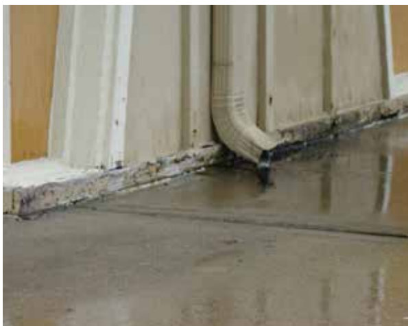
Left: The wood trim at 318 E. Highway 50 is rotted.
