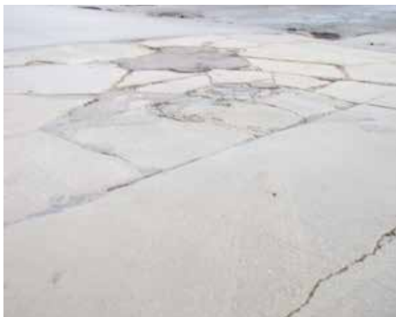
Left: The concrete pavement along E. Second Street has severe cracking.
