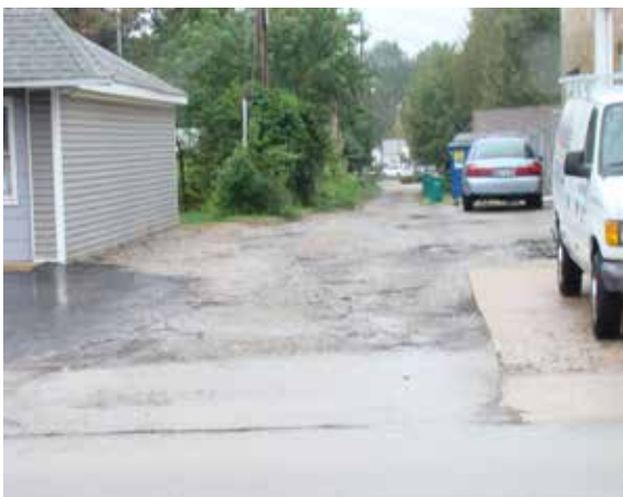
Left: A deteriorated alleyway running between Lincoln Avenue and Cherry Street.
