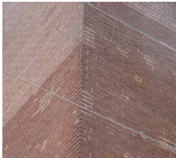
Right: The brick walls at 220 E. State Street are in need of tuck-pointing.
