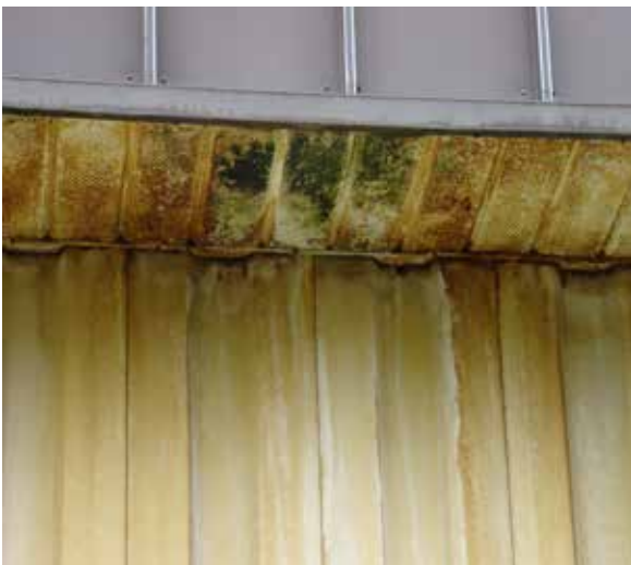
Left: Rust and algae on the enclosed soffit at 109 N. Penn Street.
