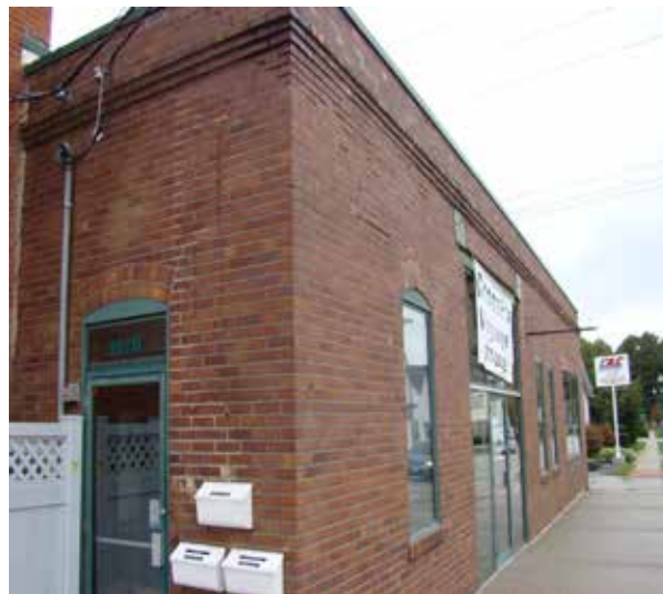
Right: The brick wall at 102 W. State Street is in need of tuck-pointing.
