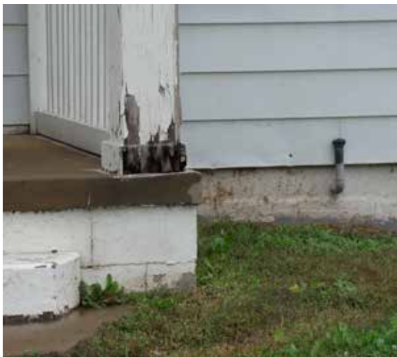
Left: A rotted wood column on the front porch of 202 W. State Street.
