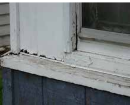
Below: The wood siding and window frame at 112 N. Lincoln Avenue are deteriorated.
