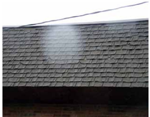
Right: The shingles on 310 E. Highway 50 are in need of replacement.
