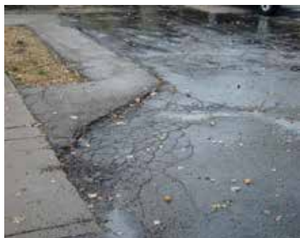
Below: The parking lot at 31 S. Lincoln Avenue is deteriorated.
