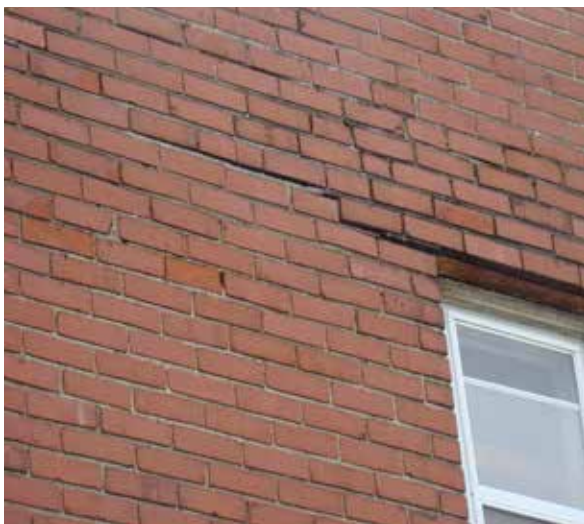
Left: The rear brick wall on 127 E. First Street is bowing outward.
