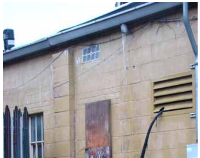
Above: A missing downspout at Southview Plaza.
