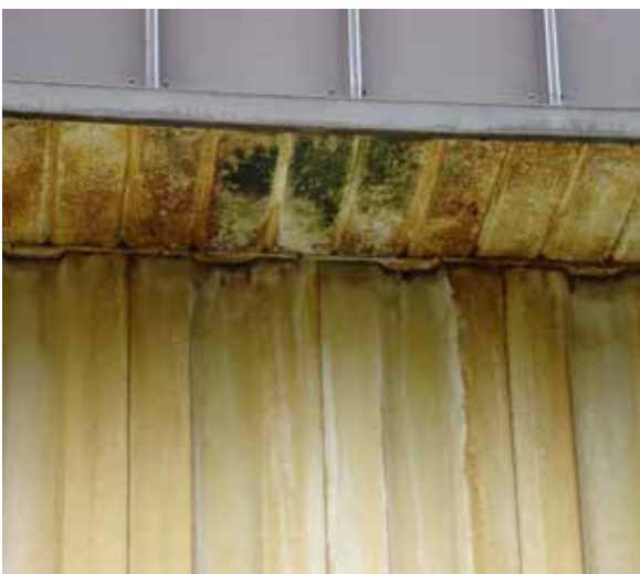
Left: Rust and algae on the enclosed soffit at 109 N. Penn Street.
