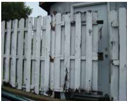
Right: A deteriorated wood fence located at 720 South Lincoln Highway.
