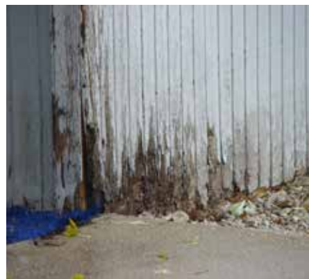
Above: Rotted wood siding on 304 S. Lincoln Avenue.
