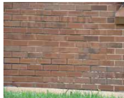
Below: 118 E. Washington Street is in need of tuck-pointing.
