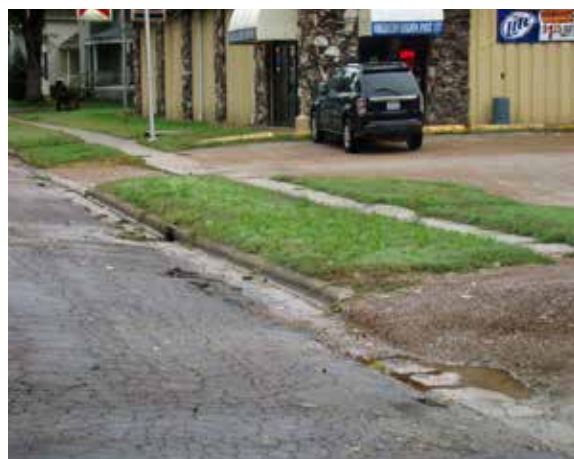
Right: E Wash- ington Street has deteriorated pave- ment and gutters.
