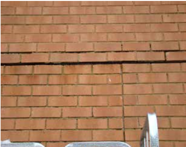
Left: Significant voids on mortar joints on the rear wall of this building in Southview Plaza.
