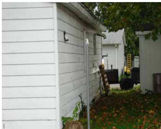
Right: Deteriorated siding at 301 E. State Street.
