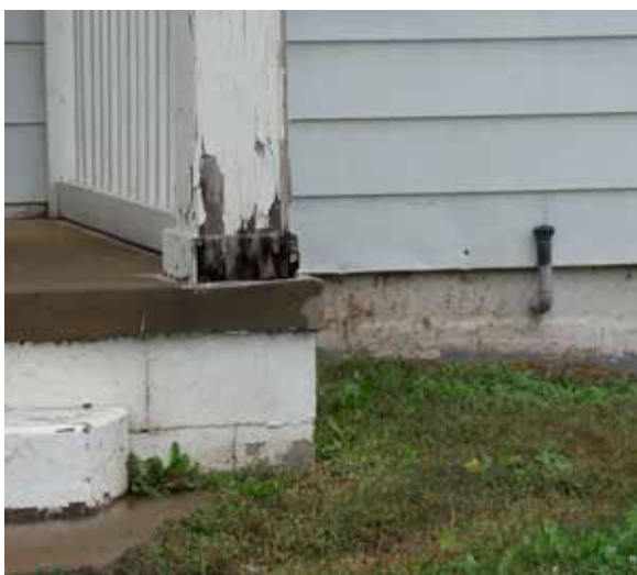
Left: A rotted wood column on the front porch of 202 W. State Street.
