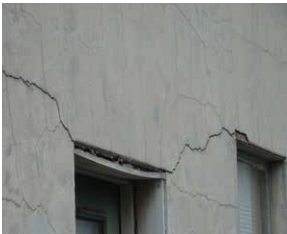
Left: The rear wall at 101 W. First Street is deteriorated.
