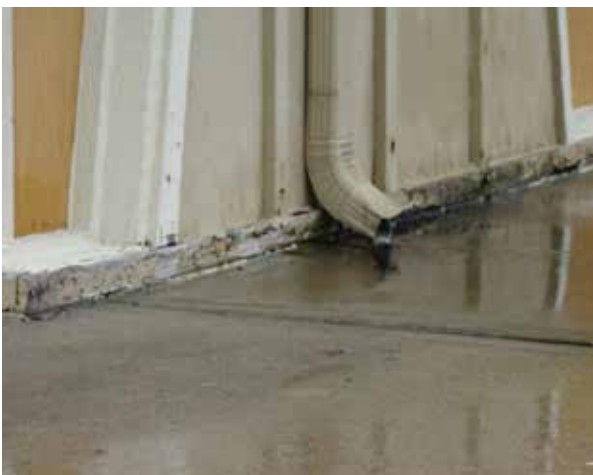
Left: The wood trim at 318 E. Highway 50 is rotted.
