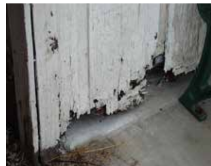
Above: Rotted wood siding at 126 E. State Street.
