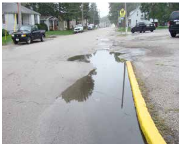
Left: The intersection of W. Fifth Street and Lincoln Avenue has deteriorated pavement and standing water due to inadequate storm drainage.
