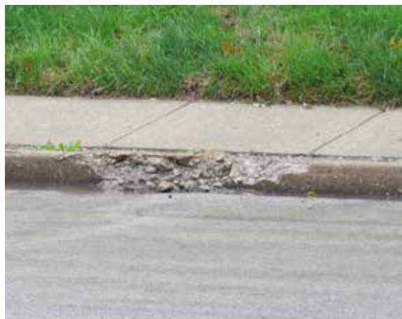
Right: Deteriorated curbing along S. Lincoln Avenue.
