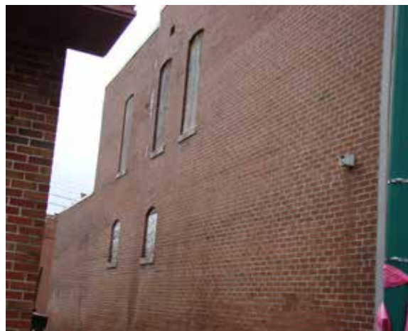
Right: 133 W. First Street has boarded up windows and is in need of tuck-pointing.
