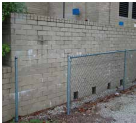
Above: the brick wall located at 502 S. Lincoln Avenue is in need of tuck-pointing.
