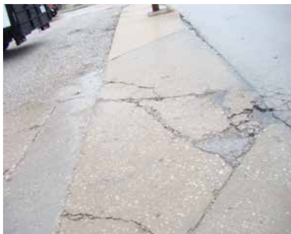
Right: A deteriorated sidewalk along Lincoln Avenue.
