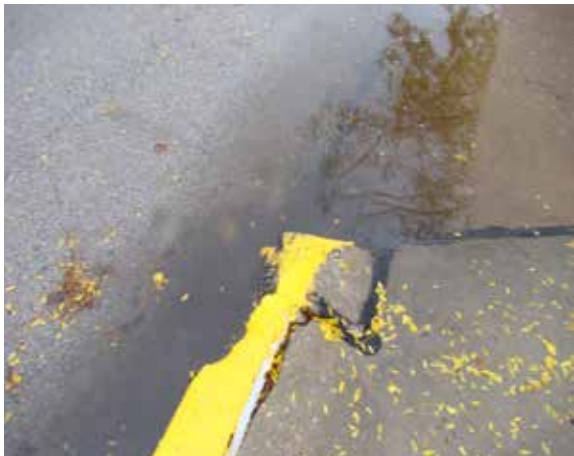
Left: Deteriorated curbing along Lincoln Avenue. Note: standing water due to inadequate storm drainage.
