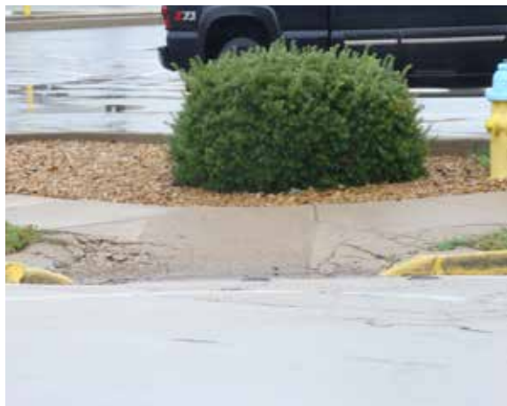
Right: A deteriorated handicap ramp located at the intersection of Lincoln and Third.
