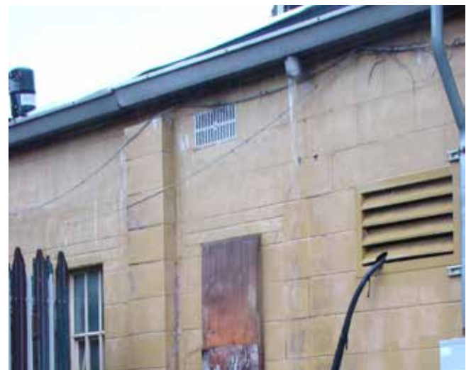
Above: A missing downspout at Southview Plaza.
