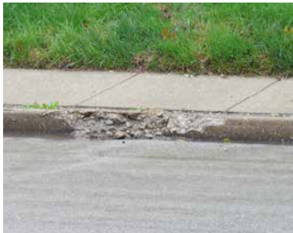
Right: Deteriorated curbing along S. Lincoln Avenue.
