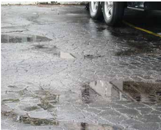
Left: The parking lot at 101 Virginia has severe alligator cracking.
