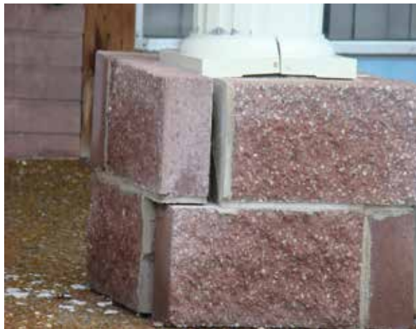
Right: The concrete block columns at Southview Plaza are dislodged.
