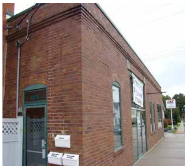
Right: The brick wall at 102 W. State Street is in need of tuck-pointing.
