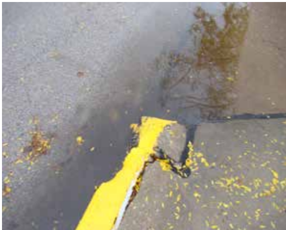
Left: Deteriorated curbing along Lincoln Avenue. Note: standing water due to inadequate storm drainage.
