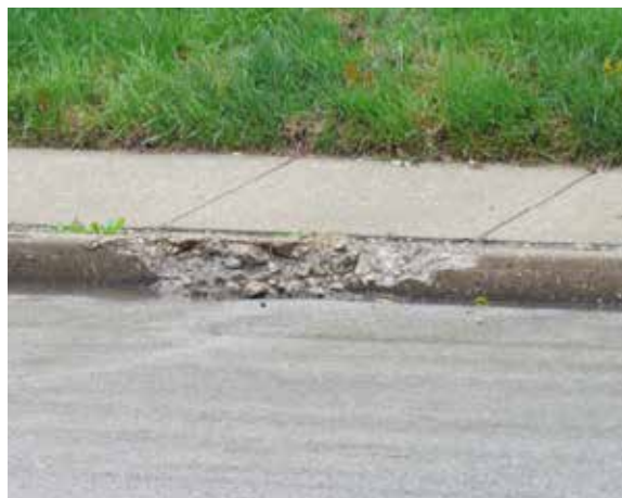
Right: Deteriorated curbing along S. Lincoln Avenue.
