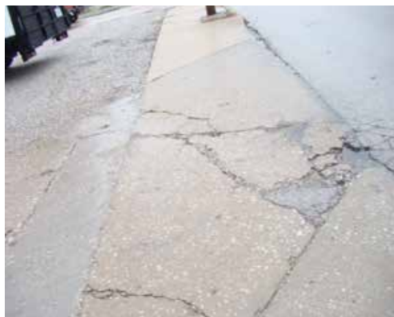
Right: A deteriorated sidewalk along Lincoln Avenue.
