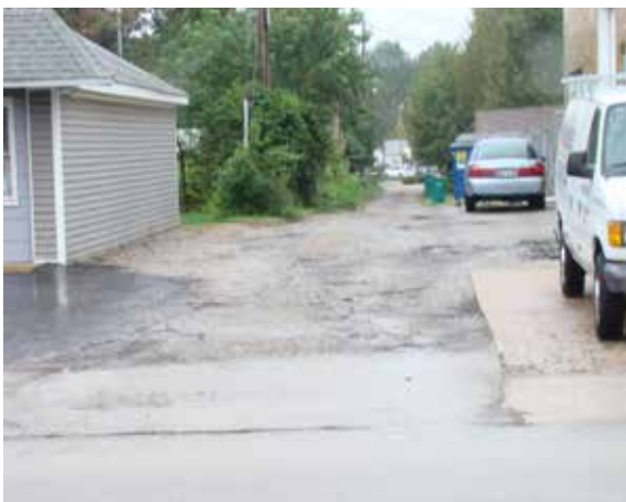
Left: A deteriorated alleyway running between Lincoln Avenue and Cherry Street.
