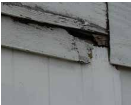
Below: Rotted wood siding at 112 N. Lincoln Avenue.
