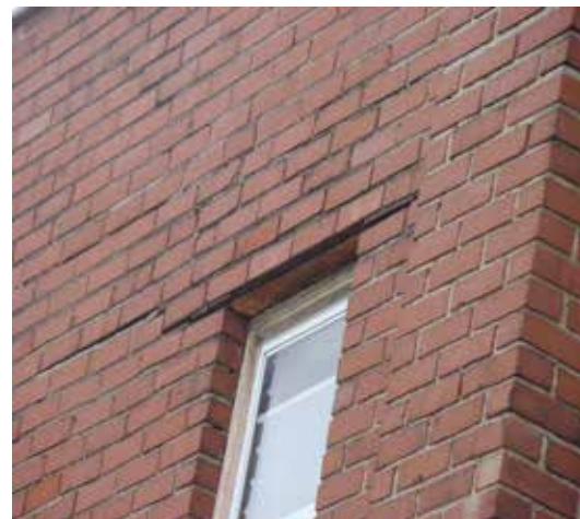
Right: A deteriorated brick wall located at 127 E. First Street.
