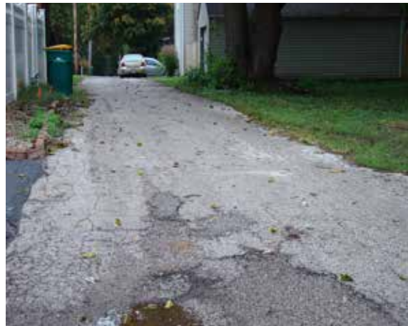
Right: This alley running between Lincoln Avenue and Cherry Street is deteriorated.
