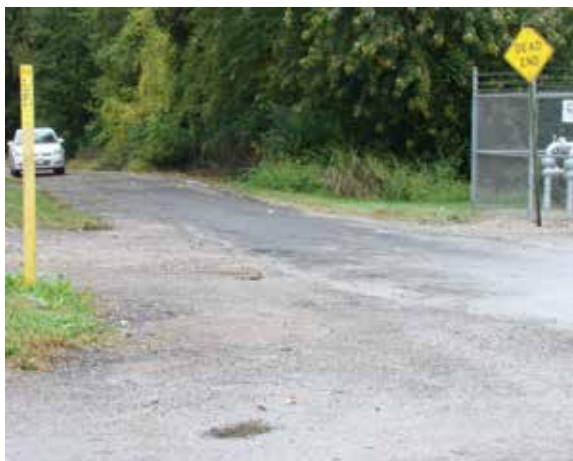
Left: Deteriorated pavements on W. First Street.
