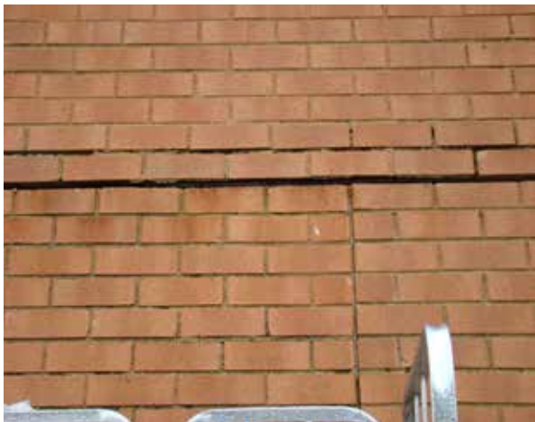
Left: Significant voids on mortar joints on the rear wall of this building in Southview Plaza.
