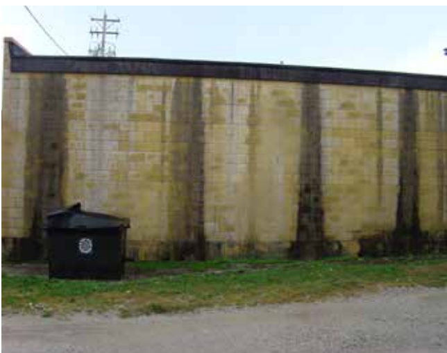
Above: Water damage to the rear of the eastern building at Southview Plaza.
