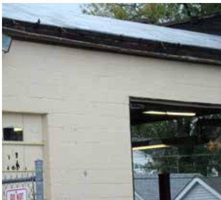
Above: Sagging gutters on 510 S. Lincoln Avenue.
