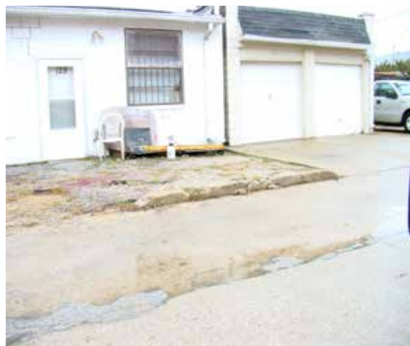
Right: Deteriorat- ed curbing along W. Second Street
