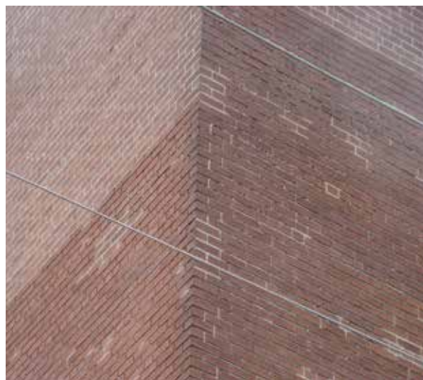
Right: The brick walls at 220 E. State Street are in need of tuck-pointing.
