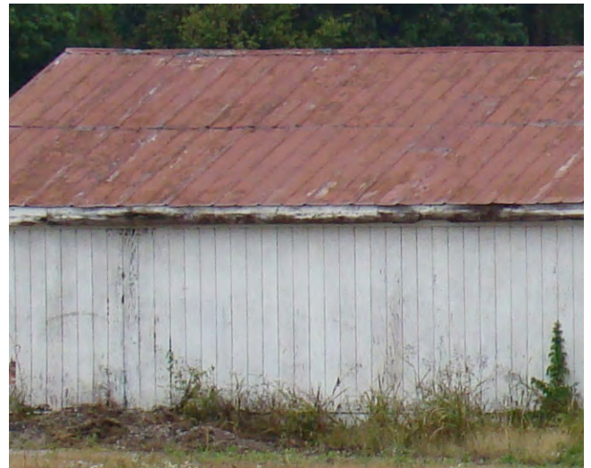
Above: The soffit and fascia at 201 Scott-Troy Road is rotted.
