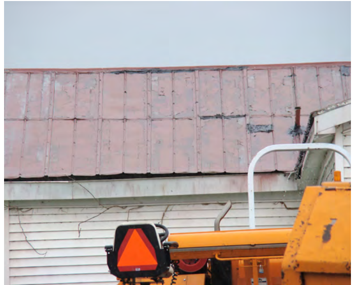
Above: The corrugated metal roof at 201 Scott-Troy Road is deteriorated.
