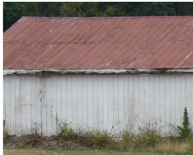
Above: The soffit and fascia at 201 Scott-Troy Road is rotted.
