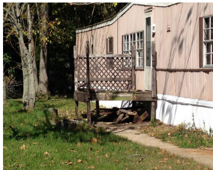
Above: A rotted wood porch on the front of one of the mobile homes at Rock Springs Estates.
