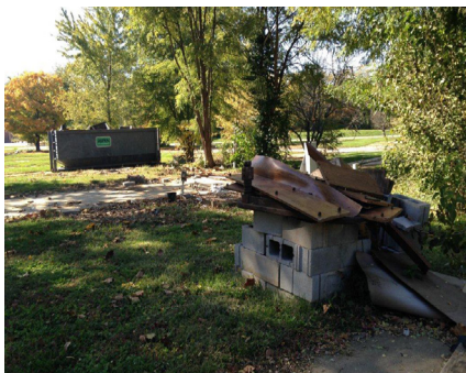
Below: Trash and debris piled on a lot next to a full construction dumpster.
