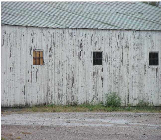
Above: The siding at 201 Scott-Troy Road has rotted.
